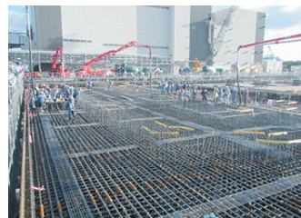
A view of massive concrete placement in the construction of foundations for Unit 3 at the Noshiro Thermal Power Station
