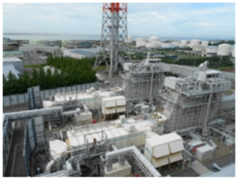
Actions to verify mixed burning of hydrogen at Niigata Thermal Power Station
