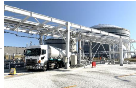
LNG shipping facility at New Sendai Thermal Power Plant
