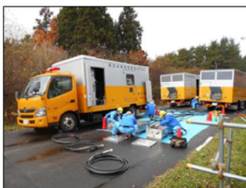
Power supply training with power supply vehicles
