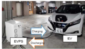
V2G demonstration project in cooperation with Nissan Motor Corporation, Mitsui & Co., Ltd., and Mitsubishi Estate Co., Ltd.
