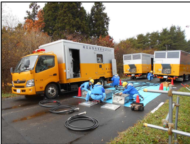
Power supply training with power supply vehicles
