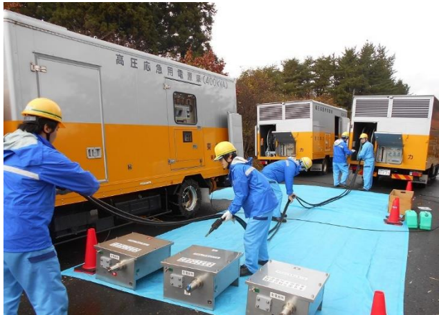
Power supply securing training by power supply car
