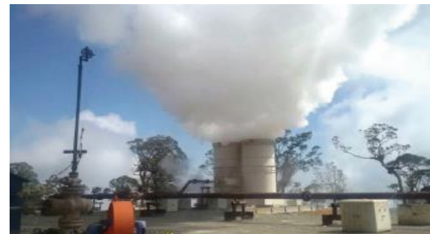
Steam power testing (Site of Rantau Dedap Geothermal Power Plant)
