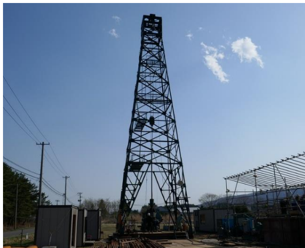
Supplementary survey (Boring geological survey : collect the soil in the deep underground and check the condition of geology directly)
