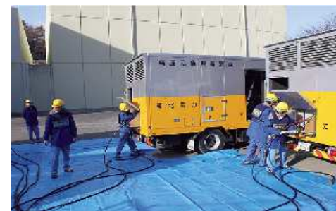
Drill in securing power resources by connecting a power supply vehicle (Onagawa)
