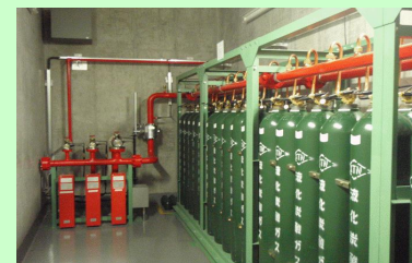
Automatic extinguishment equipment
