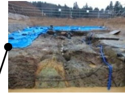
Survey on the horizontal drilling surface The points just above the faults and surrounding areas were closely inspected. No traces of strike-slip fault activity were confirmed.
