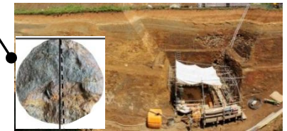
Boring survey and core cross section It was confirmed that the protrusions in the terrain are not attributed to strike-slip fault activity.
