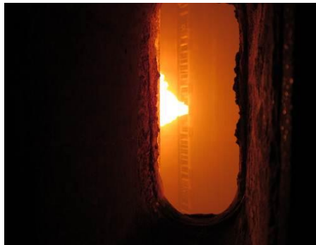
Ignition to the boiler
