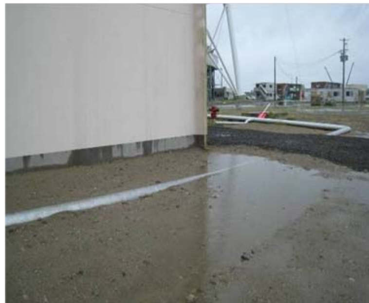
Fuel pump chamber
