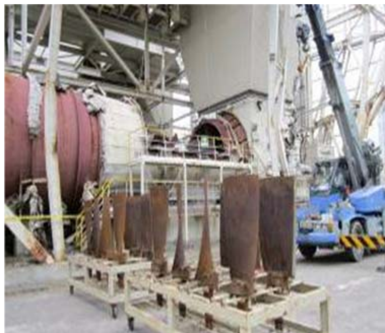
Around the boiler fan of Unit 1
