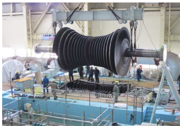
Check of Steam turbine Unit No.2
