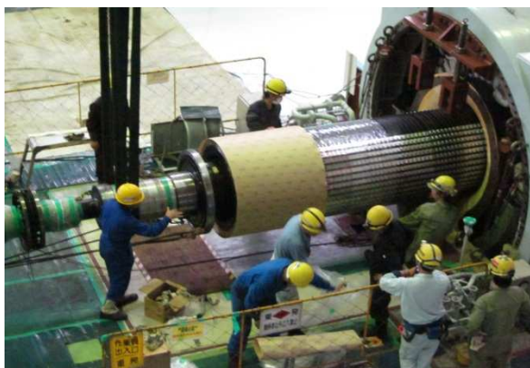
Check of Dynamo Unit No.1
