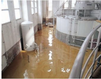
Before restoration Inundated generator room (Inundation level: 188 cm max.)
