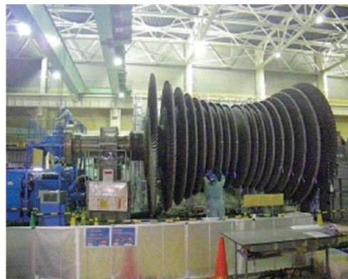
The steam turbine of Onagawa Nuclear Power unit 2 opened for inspection. (In September, 2011)
