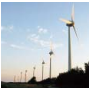
Noshiro Wind Park (14,400kW) Tohokushizen-e.co.jp Tohoku EPCO Group
