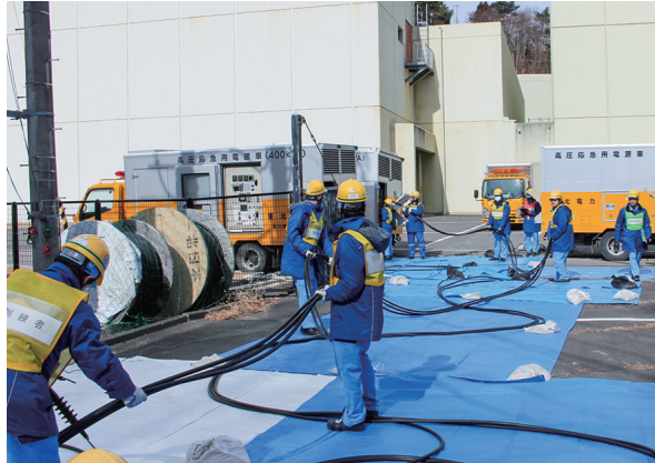
Training on connecting cables to a power supply vehicle for emergency power supply to the power station (Onagawa Nuclear Power Station)
