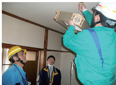
Towada Network Center performs electric facility inspections and cleanup activities for elderly single-person households.
