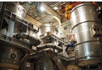
Container ventilation equipment equipped with filters
