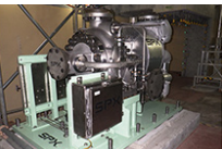
High-pressure alternative water injection equipment
