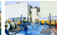
Drill involving use of mobile power generators to supply power (Onagawa Nuclear Power Plant)
