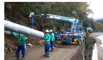
Power distribution recovery work on a temporary road built by the Japan Self-Defense Forces
