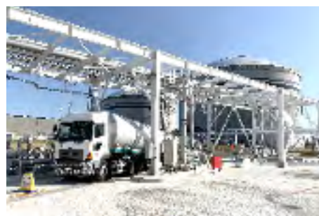
LNG shipping facilities for the Shin-Sendai Thermal Power Plant
