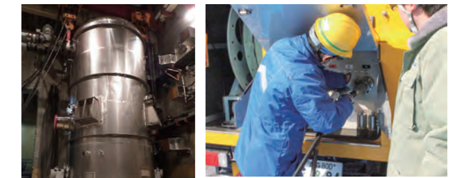
Training in connecting a power supply car to carry electricity to the nuclear reactor building (the Higashidori Nuclear Power Station)
