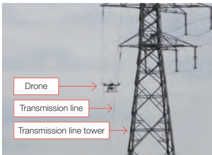
We are evaluating labor saving by using drones in transmission line maintenances and construction work.
