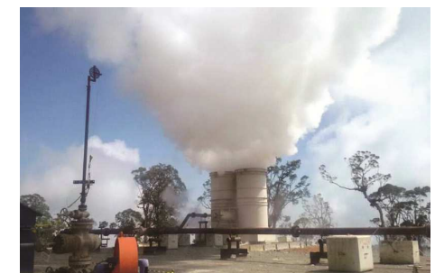
Rantau Dedap geothermal power generation project, scheduled to start commercial operation in the second half of 2020 for which construction is currently under way.
