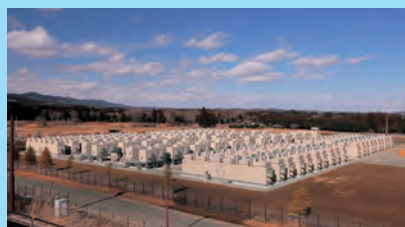
Minami Soma Substation Storage Battery System
