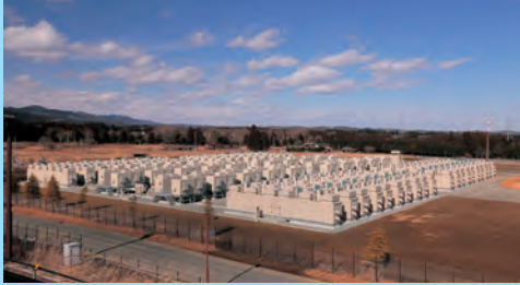
Minami Soma Substation Storage Battery System
