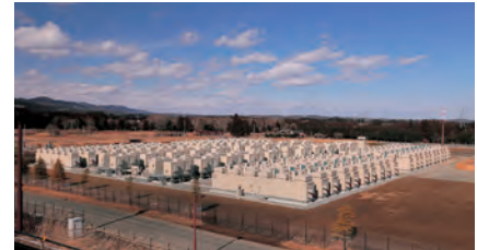
Minami Soma Substation Storage Battery System
