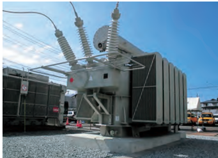
New distribution transformer
