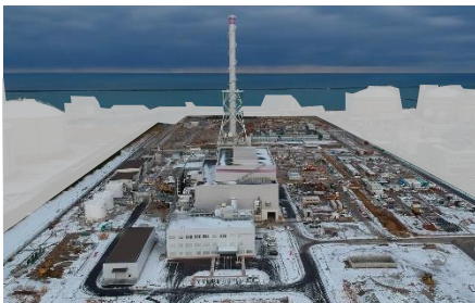
Progress of construction at Joetsu Thermal Power Station Unit No. 1 (as of January 2022)
