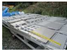
N5_鋼製架台(1)
